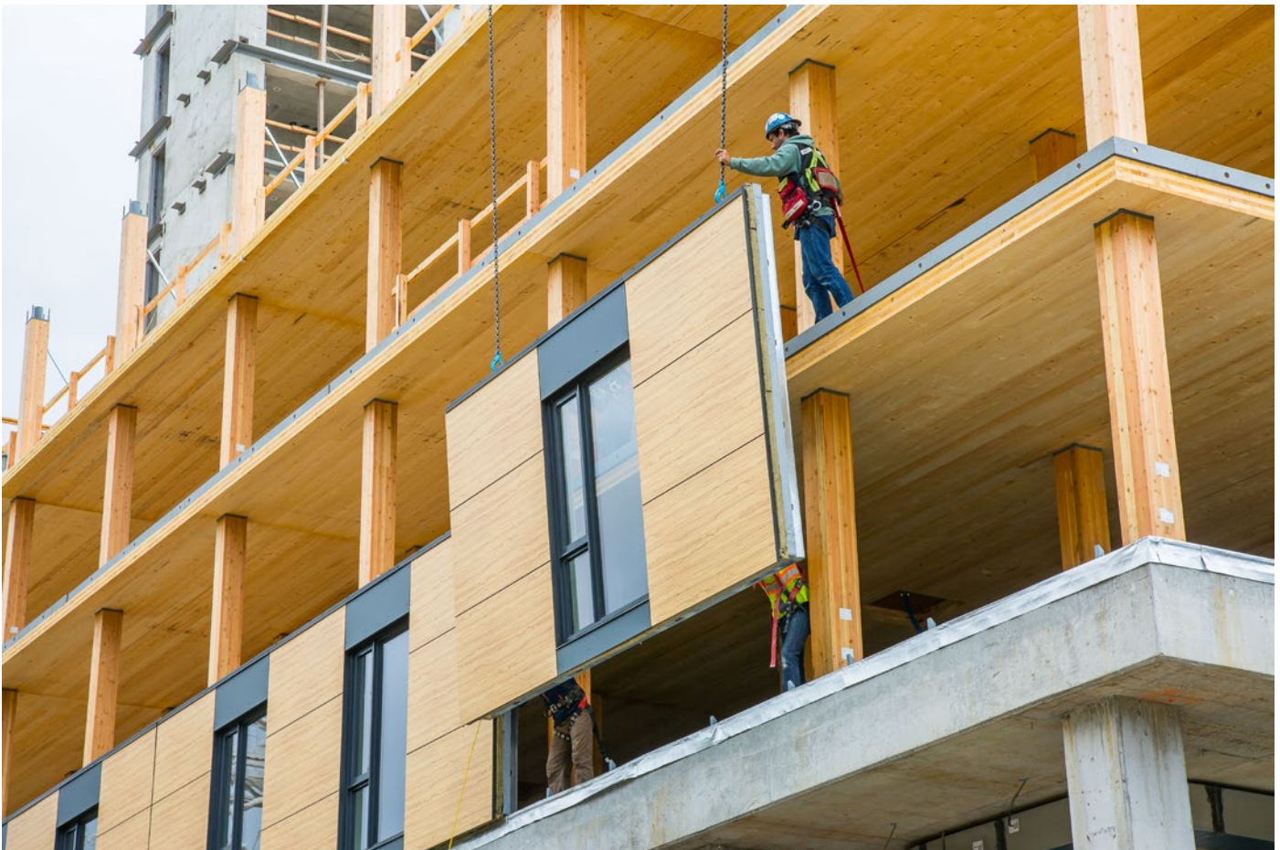
Figure 1: Tall wood innovation. One example of innovative building technology. The University of British Columbia Brock Commons mass timber building located in Vancouver is shown when it was under construction. It is now completed and – at 18 storeys – is currently the world’s tallest timber building. Photo credit: KK Law / naturallywood.com
